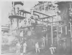
Metal tradesmen working at various levels at the Heavy Vacuum Gas Oil Hydrodesulfurization Unit 26 (D2AR).
